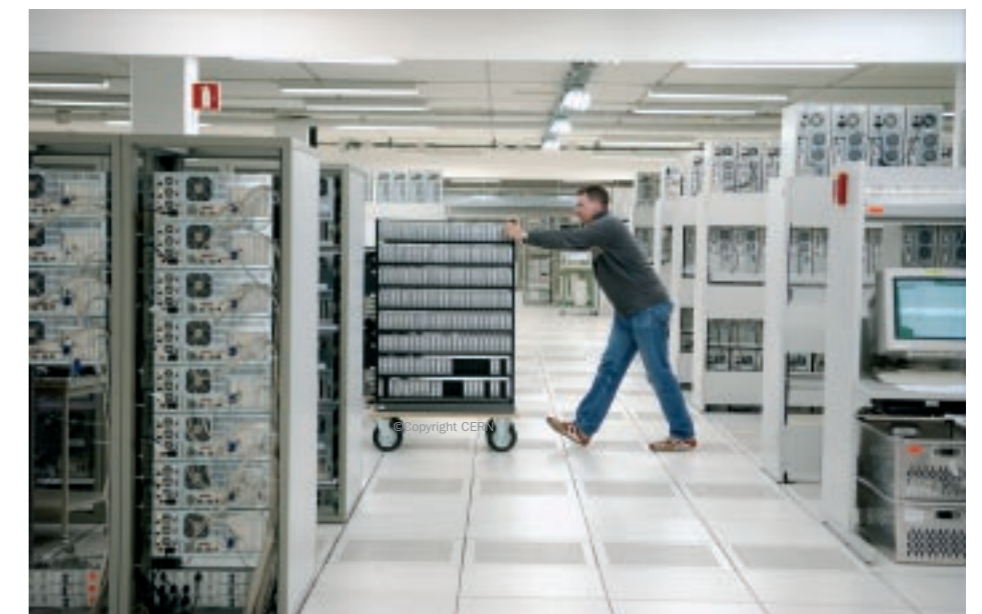
CERN data centre
