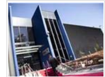
Photos: Macquarie Telecom's Intellicentre 2 Sep 24, 2012 (13 images)
