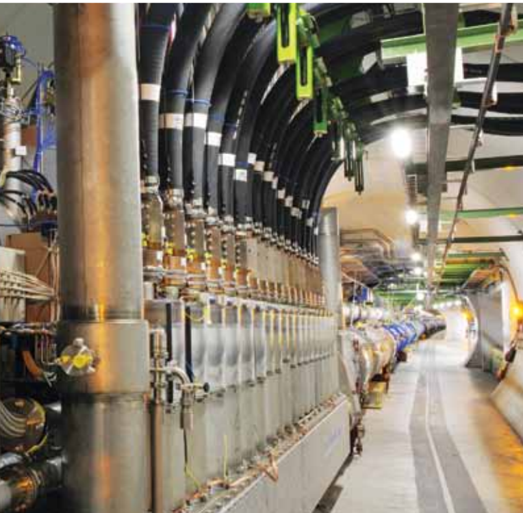
Cryogenic installation in the LHC tunnel controlled by Siemens automation equipment.
