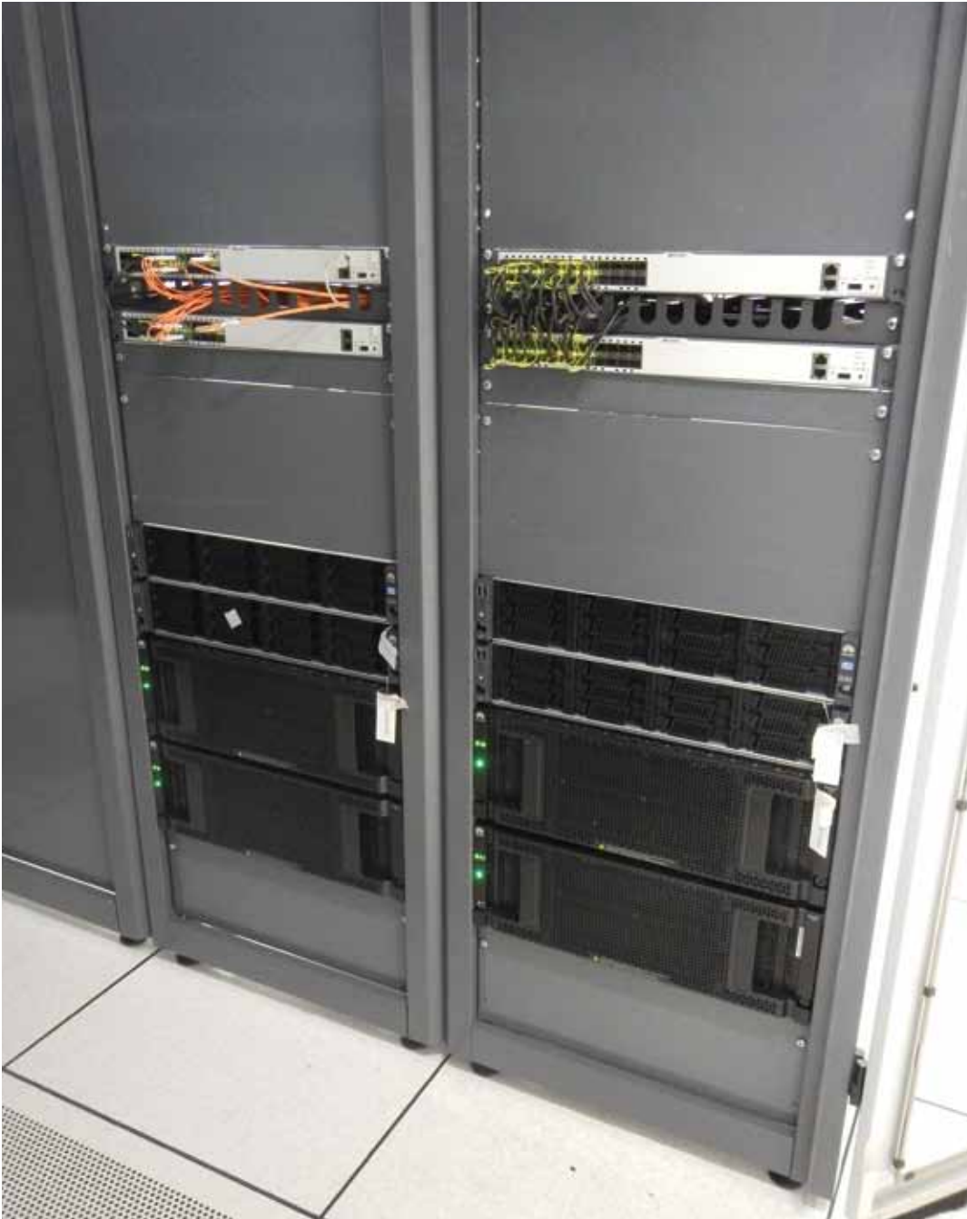
Second Huawei cloud storage setup in the CERN data centre.
